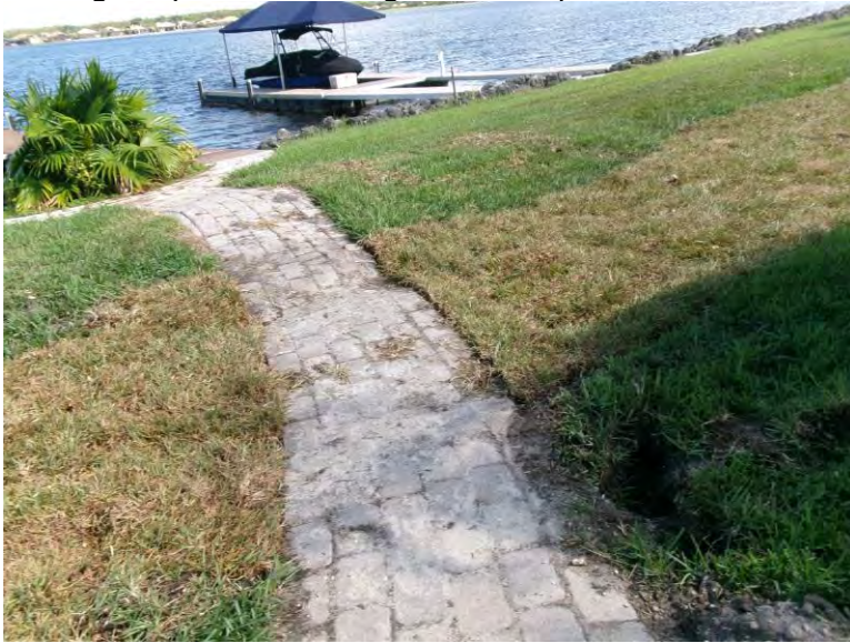
Damage to pavers crossing skid steer path
